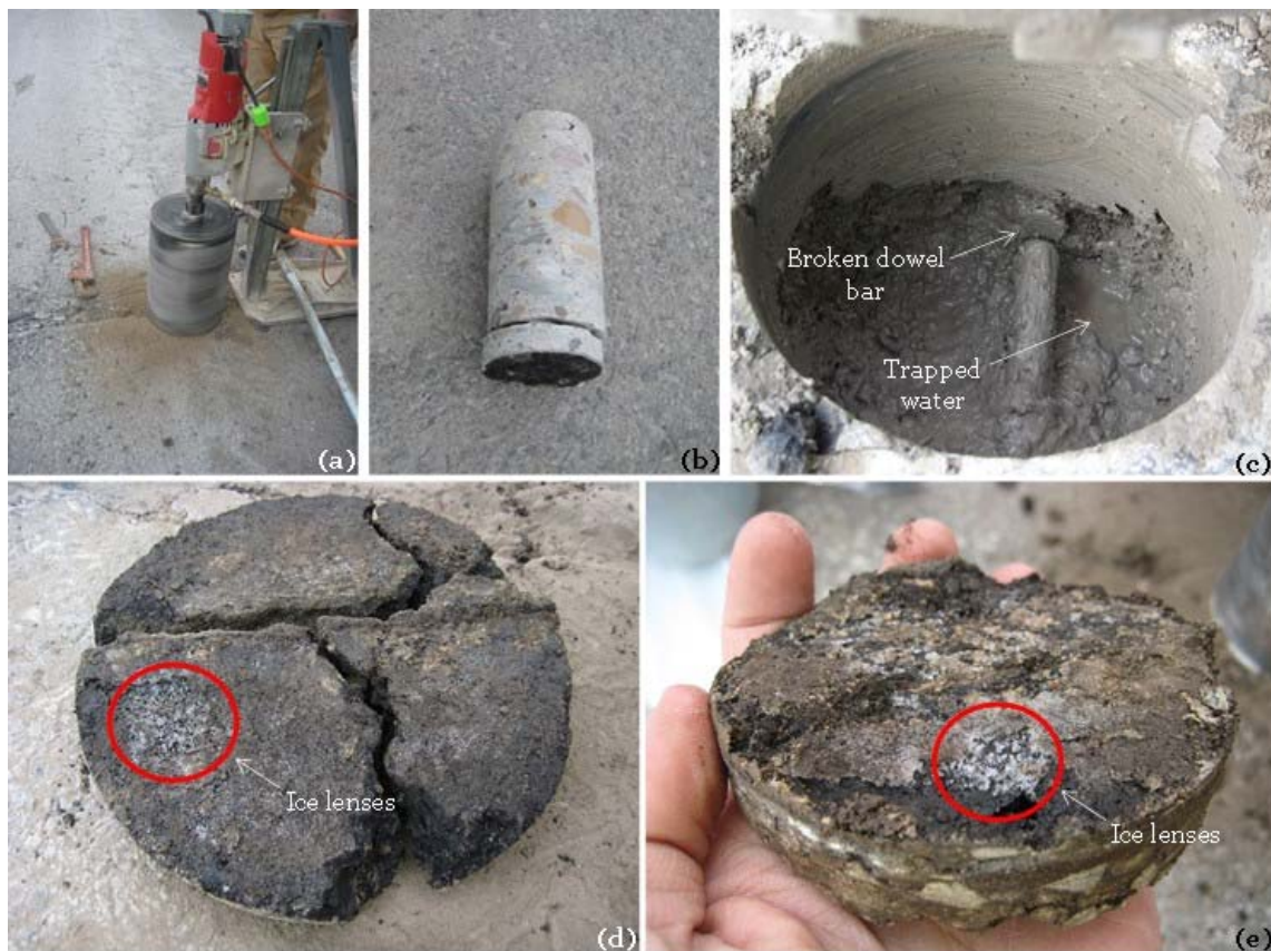
Figure 4.2. Core extraction and inspection: (a) drilling core from pavement surface, (b) subsurface concrete specimen, (c) holes with trapped water, (d) broken asphalt concrete specimen, and (e) presented ice lenses.
