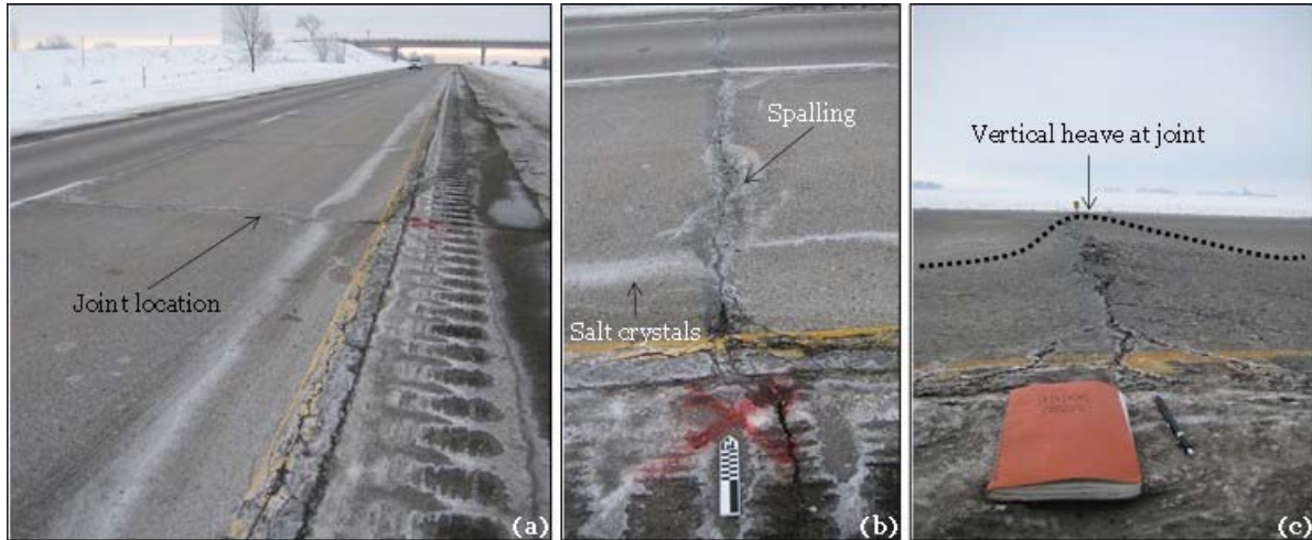
Figure 4.1. Field pictures showing (a) the EB on US 30, (b) joint deterioration with spalling, and (c) vertical heave at joint location.
